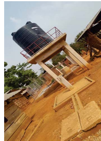
Community Solar Powered Water System, Bredi, Ahafo Ano North Municipal, Ashanti Region
