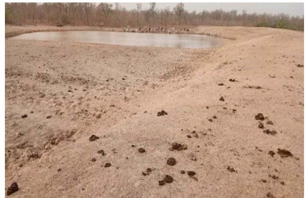
Small earth dam at Lampoga in the Bole Bamboi Constituency, Savannah Region
